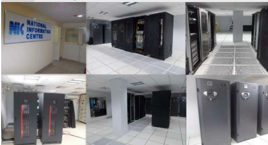
▼ Fig 2.5 NIC West Bengal State Data Centre
